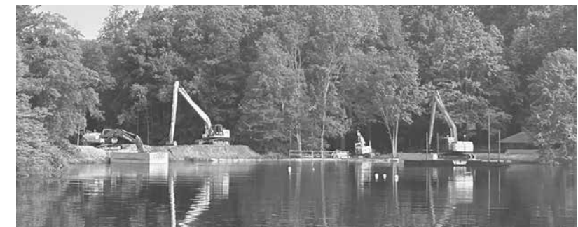
Representative Poulos secured a $500,000 DEEP grant to finish the dredging of Sloper Pond.
